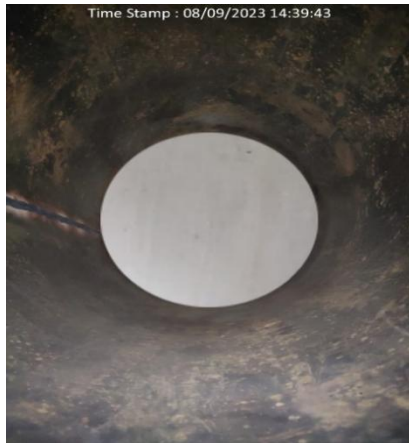
Fig 6.2 a): Image of Good pipe
