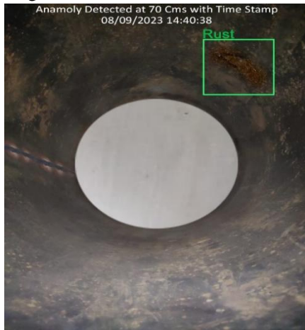
Fig 6.2.1 a): Image of rust in Pipe
