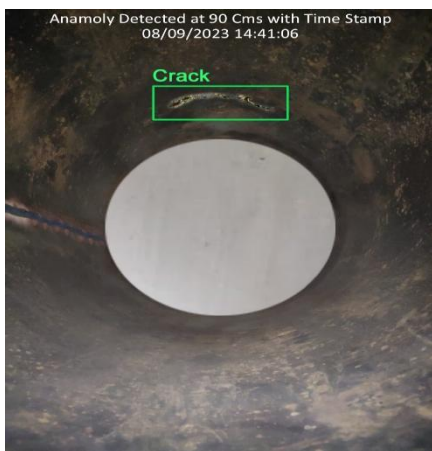
Fig 6.2.2 a): Image of crack in Pipe
