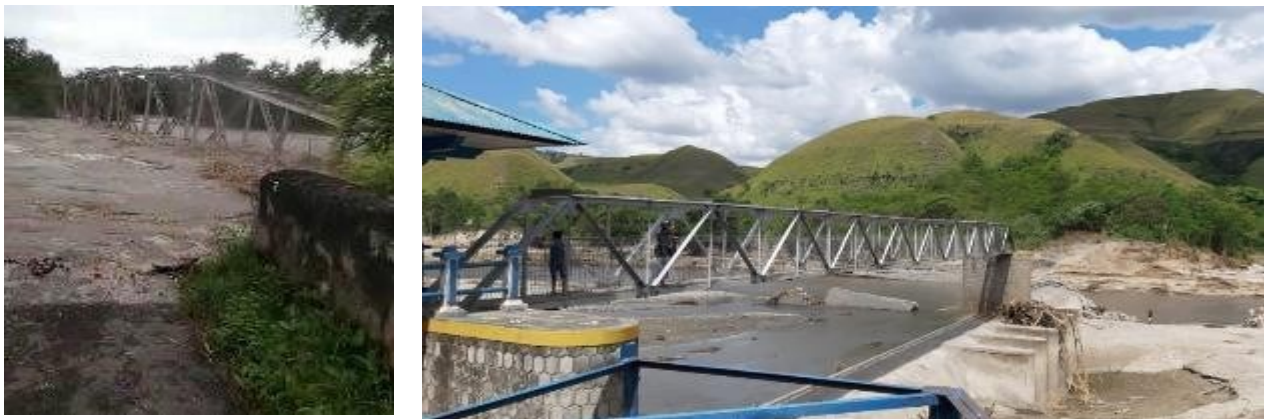
Figure 1. The collapse of the Kambaniru Bridge due to Tropical Cyclone Seroja
